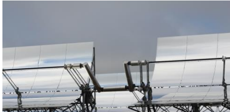
Clean Technology and Energy
